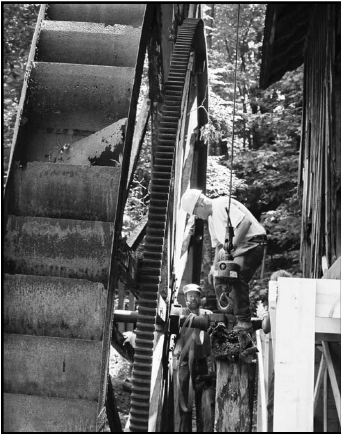
Lou Mogavero and Will Hines attach the boom crane cable to the wheel before it is lifted from its precarious angle and gently set back down on a new, temporary support. Photo by Jamie Donahoe
